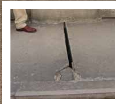
TWO VIEWS EAST ACROSS BRIDGE DECK AND SIDEWALK (inset) Expansion joint in sidewalk and bridge deck condition.
