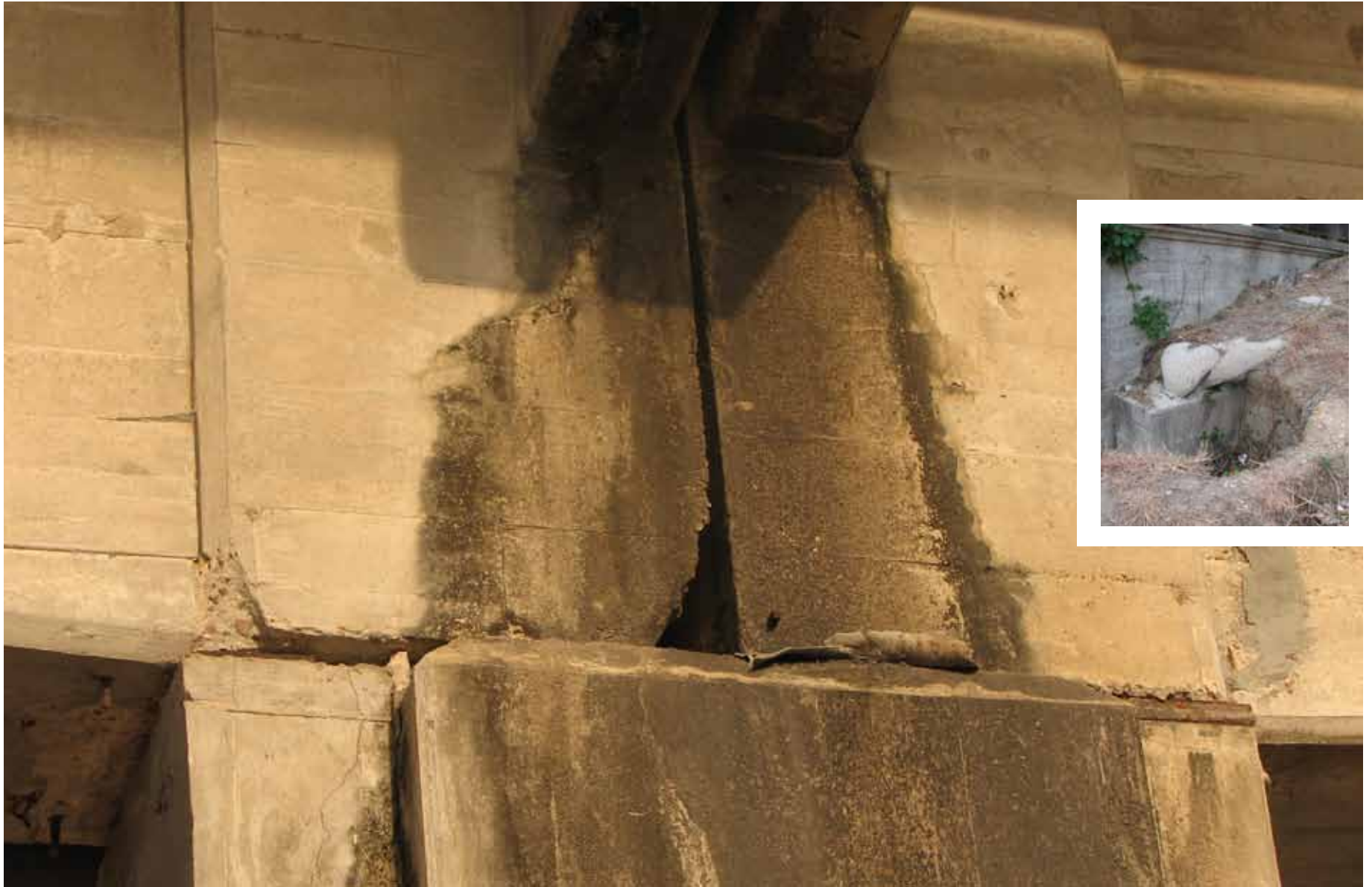
VIEW AT WEST PILING & BRIDGE BANK (inset) Floodwater impacts.
